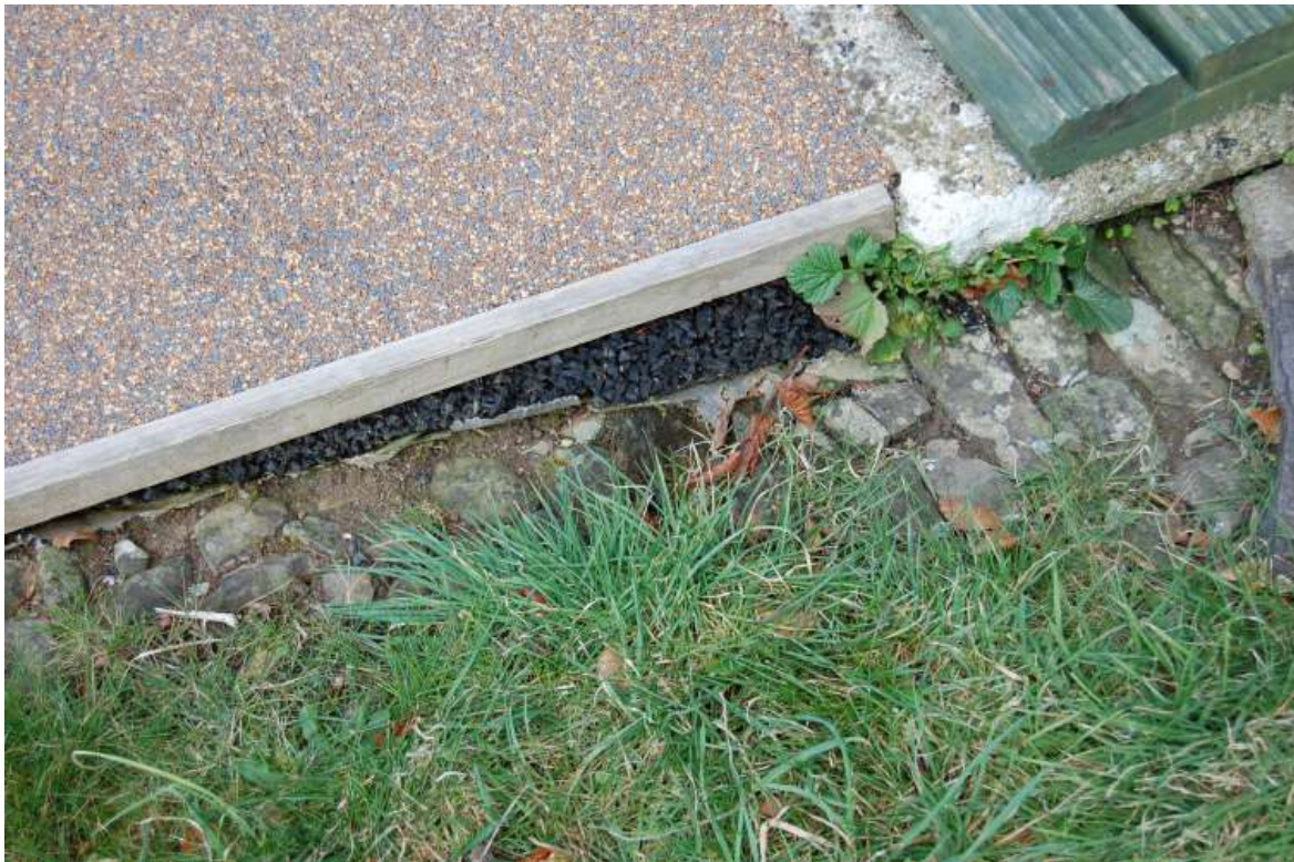
Fig.26. A detail showing the system for covering the old cobbled path. Peter Marlow.
