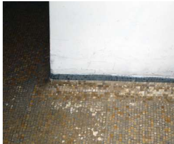
Fig.20. The mosaic flooring in the corridor and entrance hall curves up the wall for easy cleaning. Keystone, 2012.
