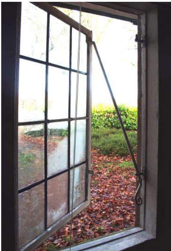
Fig.21. Voysey's ingenious vertical window stays allow for two open positions for the windows. Keystone, 2012.
