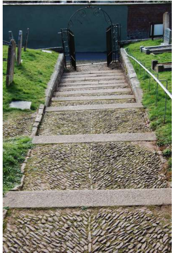
Fig.8. Cobbled steps to the Church of St Swithun, Sandford: cobbles trimmed with granite treads and laid diagonally to carry rainwater off to the sides. Peter Marlow.
